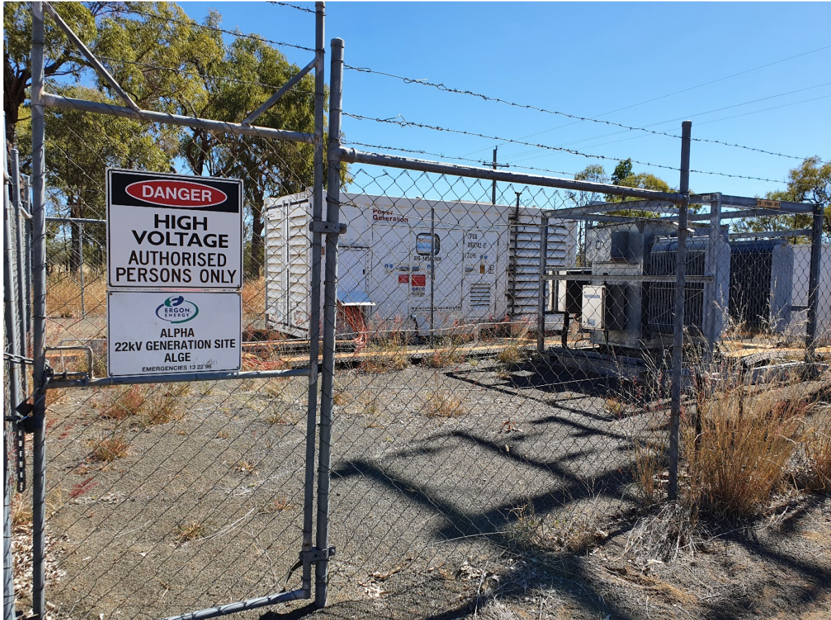
Figure 4: Standby generator connected to the Alpha 22 kV system 4
